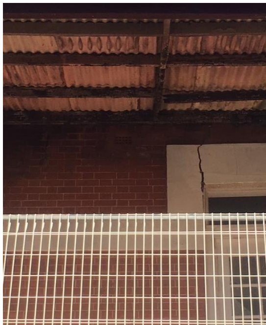
Image 2: Cracking of Brickwork Window 2 nd Storey, Matong Street Frontage
