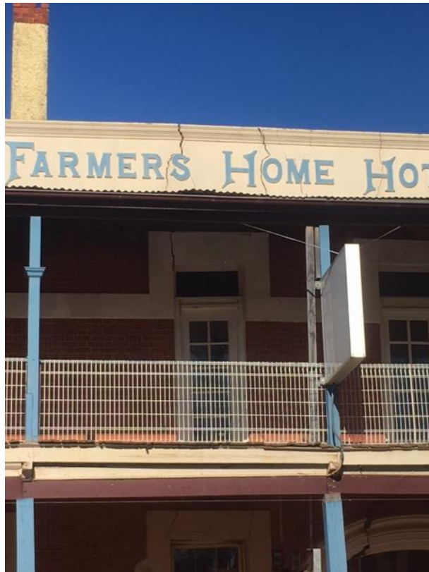
Image 3: Cracking of Parapet, Matong Street Frontage
