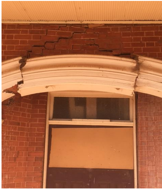
Image 1: Cracking of Brickwork Window, Matong Street Frontage
