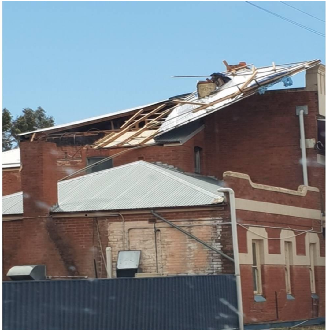
Image 1: Roof Damage after wind event
