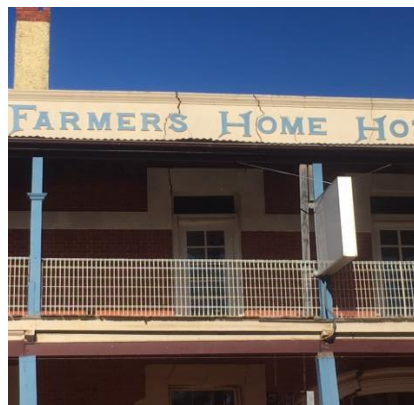
Image 3: Cracking of Parapet, Matong Street Frontage
