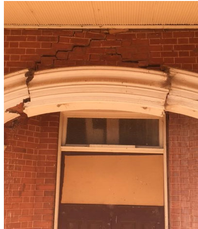
Image 1: Cracking of Brickwork Window, Matong Street Frontage
